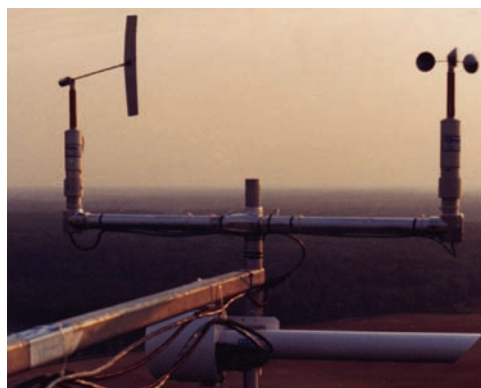
Anemometer, vane and air temperature instrument cluster mounted on extendable boom at 100m level of tower installed and operated by Enviroplan Consulting in Dinwiddie County, VA.
